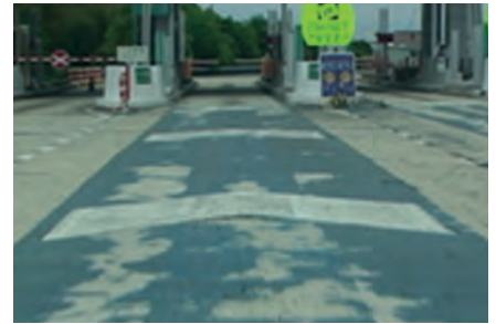
Epoxy markings after 1 year
